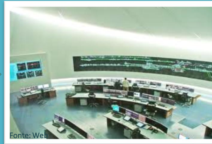
Centro de Controle Regional
